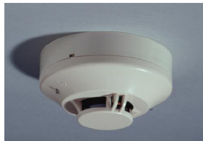
B501 Base Installed with Detector
